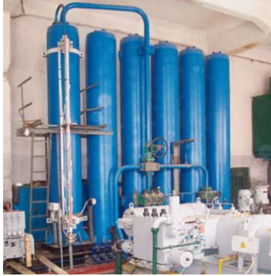
Accumulator station – HELWANT, Egypt
